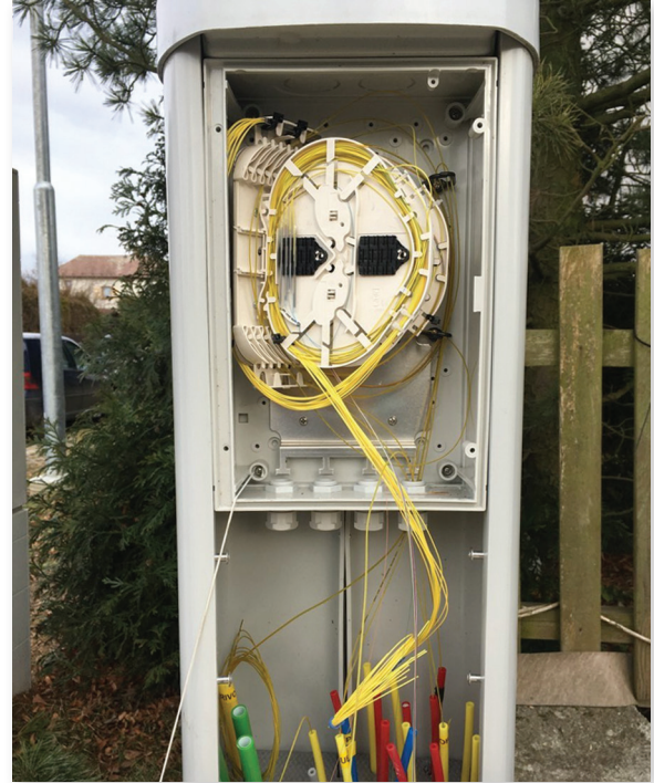
Fiber distribution point
